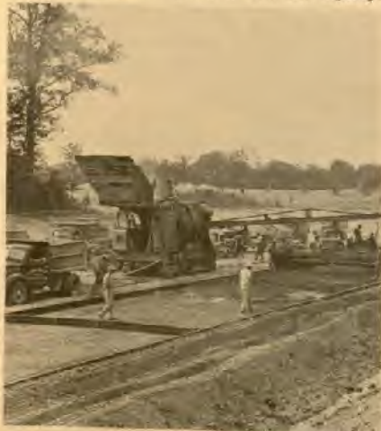
In the late 1940s, construction workers built Virginia's first expressway—the Shirley Highway in the northern part of the state.
