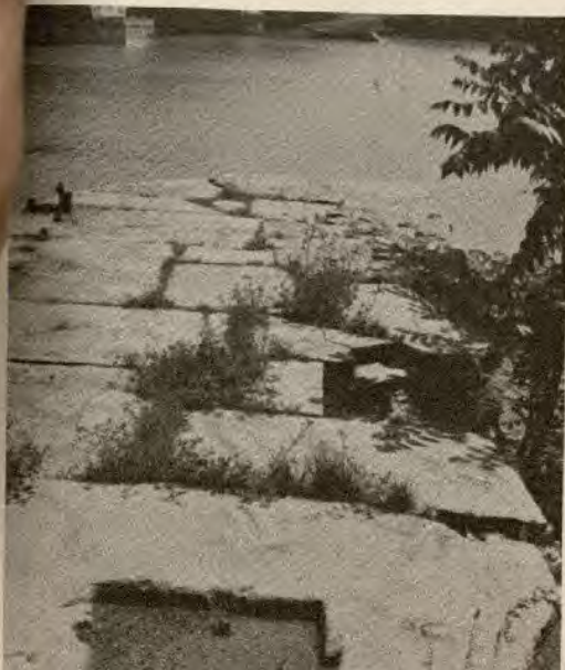
Top of North Abutment and tow path looking towards Virginia across the Potomac with all that remains of the last visible pier, near
