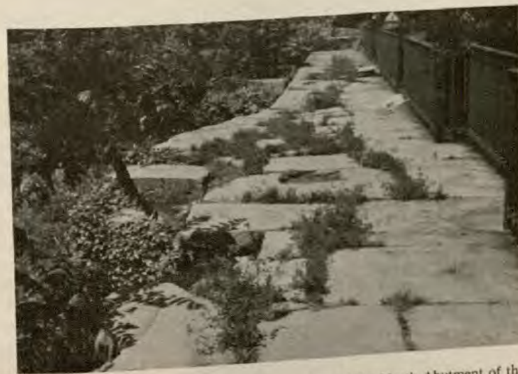
Top of the North Abutment of the Alexandria Canal with edge of Turning Basin and unloading slip, looking northward towards the Chesapeake and Ohio Canal.
