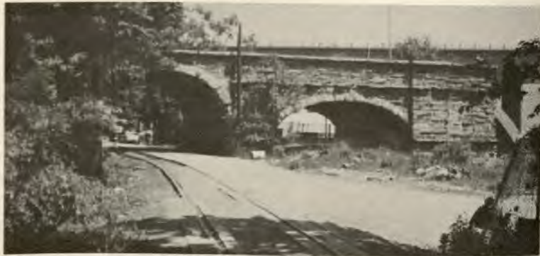
North Abutment of the Alexandria Canal showing the vehicular arch with railroad passing through.
