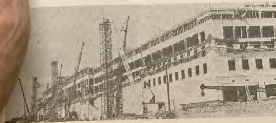
SC 647819 Construction of the Fifth Floor and the Bus and Taxi Entrances.
